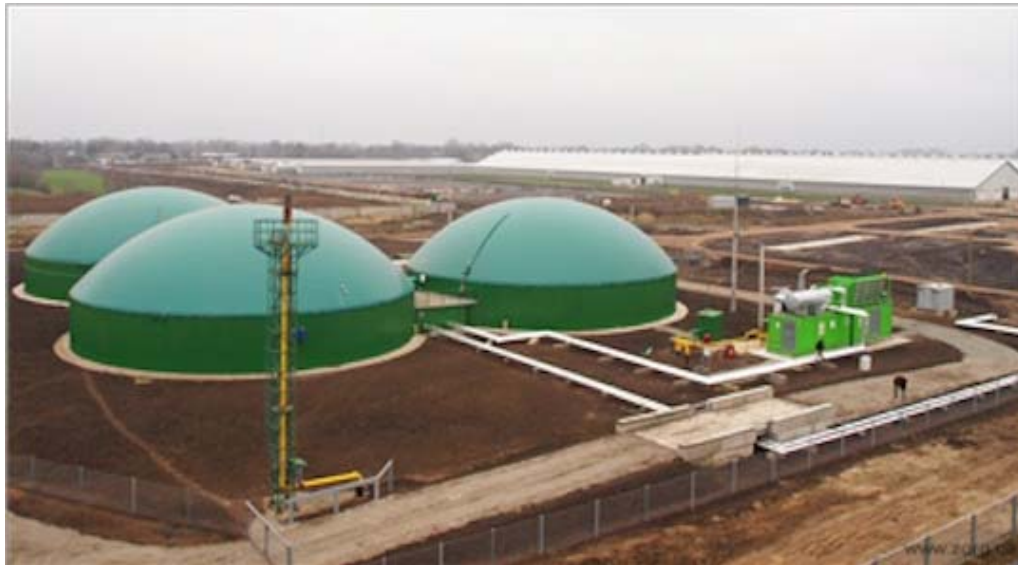
Figure 8: Enclosed Bio Gas Tanks
