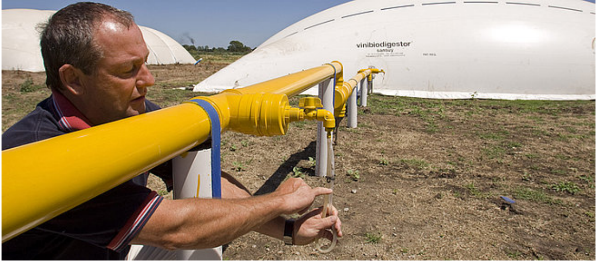
Figure 9: Bio Gas Pond with Tent Collection
